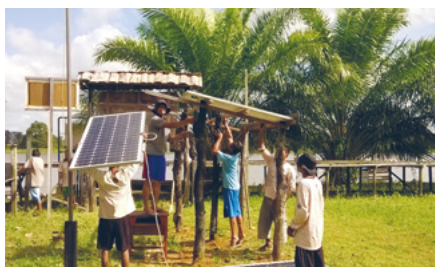
Rimba Raya funded community solar panels
